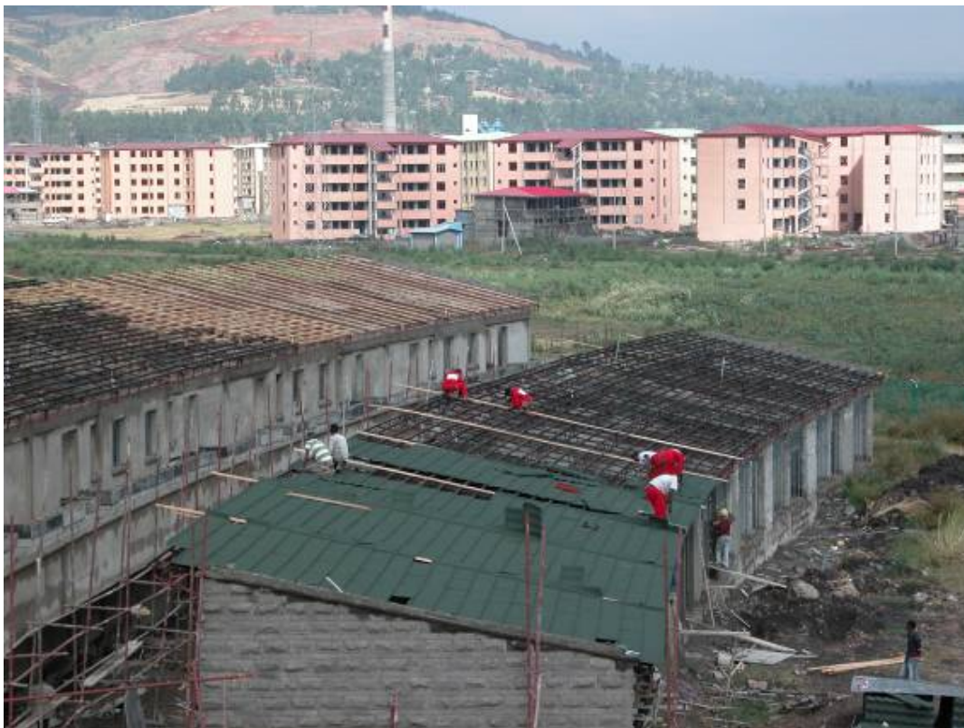
Installing the roof cladding to the Staff Residence Building. (Het aanbrengen van de dakbedekking)
