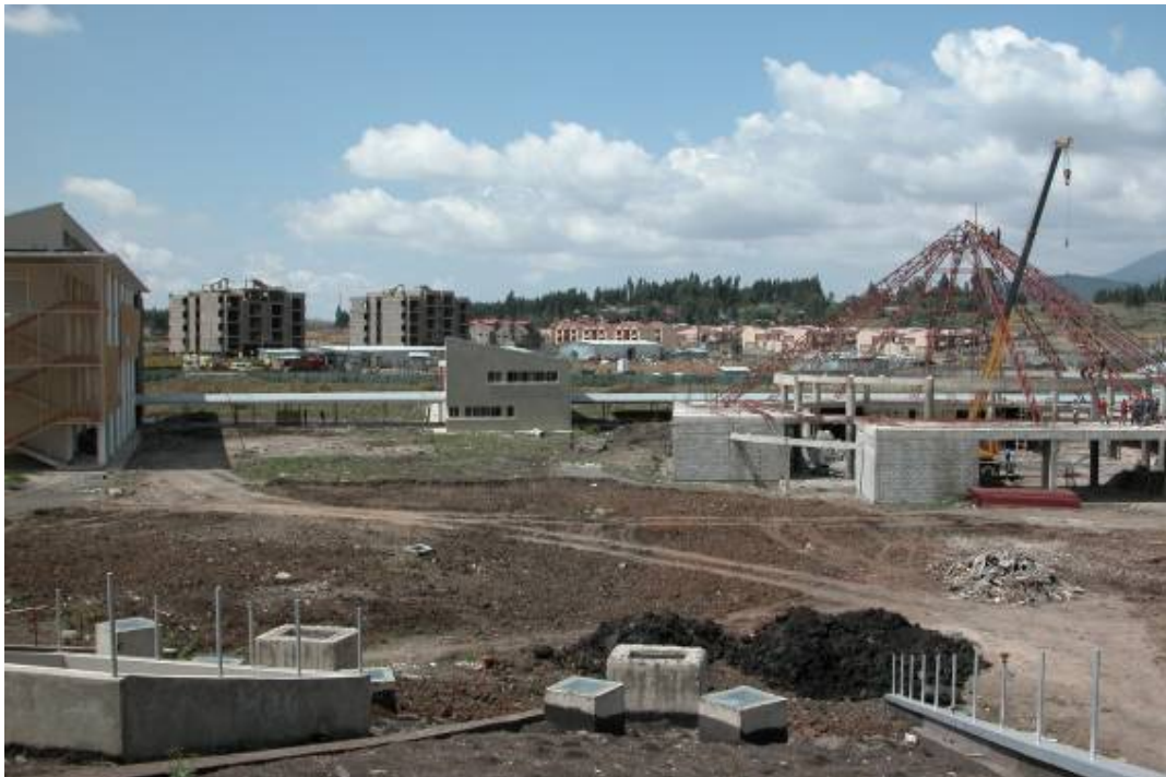
Classroom Building (B) at the left, Administration (C) in the middle, and Multi-purpose Hall (D) at the right.
