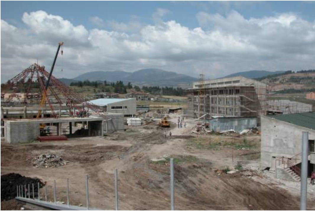
From left to right the Multi-purpose Hall (D), Faculty Office (E), Classroom Building (F), and a corner of the Staff Residence Building (H).
