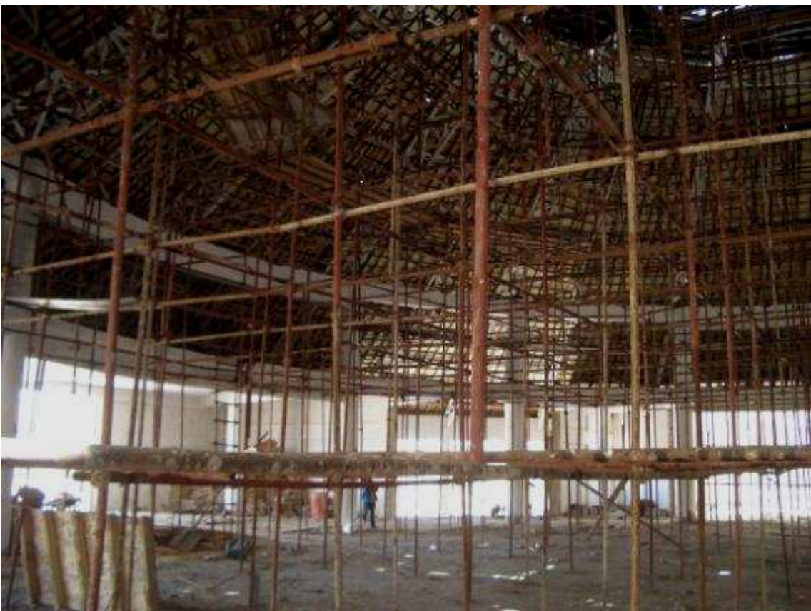
The ceiling work in the auditorium will be started after finishing the roofing.
