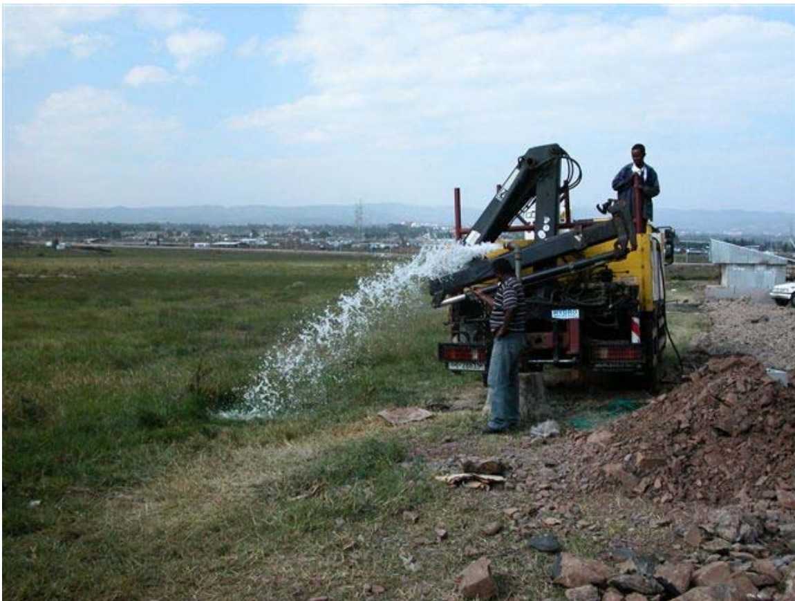
The pump has been commissioned and tested.
